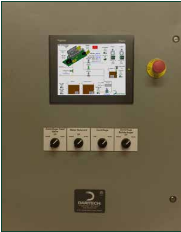
Decanter Centrifuge Control Box
